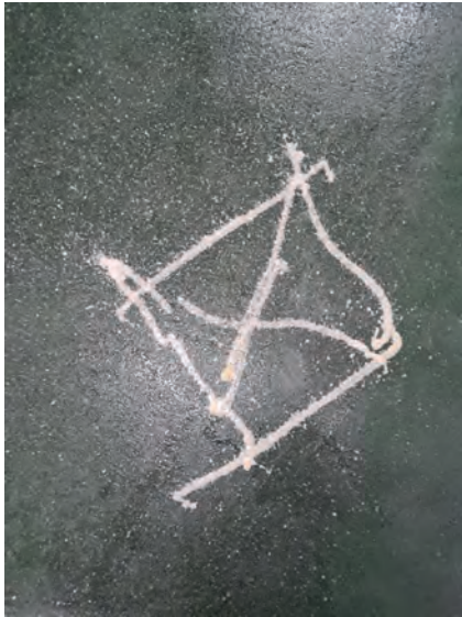
Biotector was applied to the floor and substantial biofilms were found to be present after caustic hypo foam clean.
