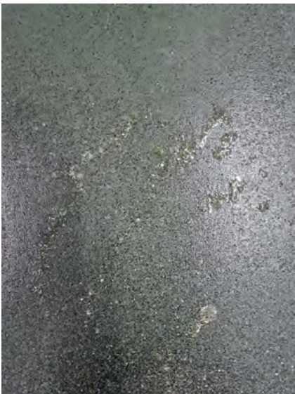
Biotector was applied to the floor and substantial biofilms were found to be present after caustic hypo foam clean.
