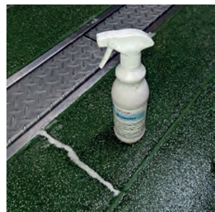
Within 5 seconds of application of Biotector biofilm is revealed in the damaged area of floor
